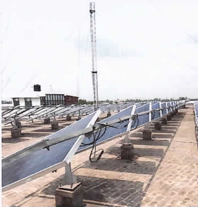
Solar Panel installed in Campus
